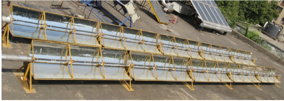
Fig. 3. Photograph of installed CPC system.
