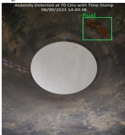
Fig 6.2.1 a): Image of rust in Pipe
