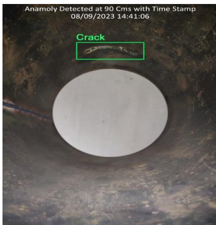
Fig 6.2.2 a): Image of crack in Pipe
