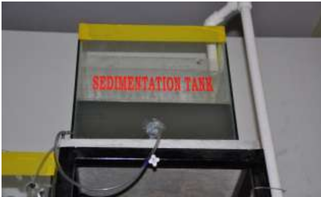
Fig.2(a):Primary Settling Unit (Sedimentation tank)
